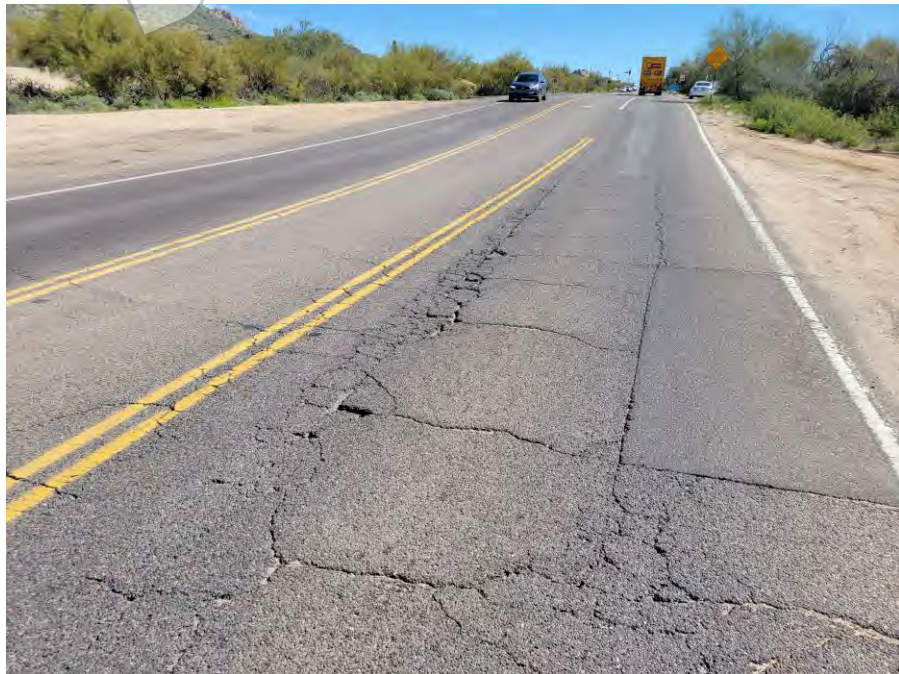
Photograph 4: Example of alligator cracking and patch in poor drainage area.
