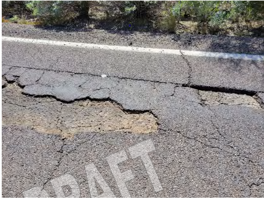
Photograph 3: Example of delamination of previous overlay
