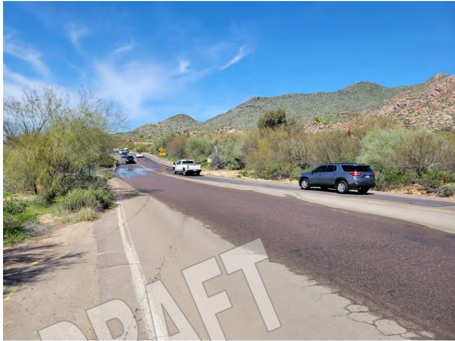
Photograph 5: Example of poor drainage.
