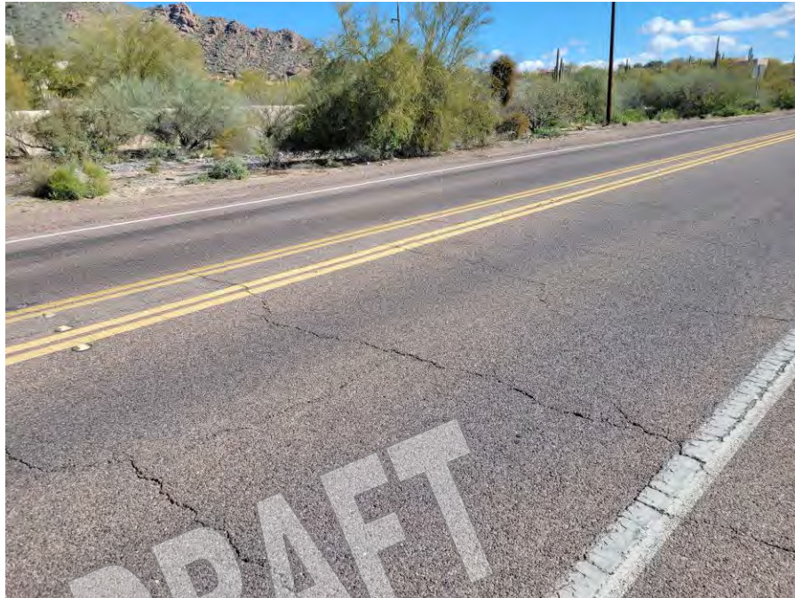
Photograph 1: Typical block cracking.
