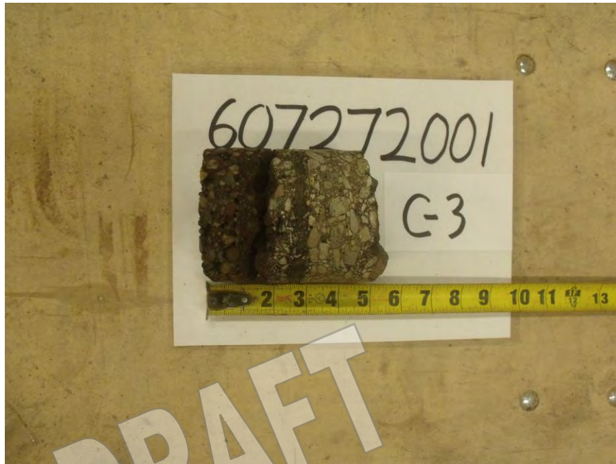
Photograph 9: Core Location C-3, asphaltic concrete thickness approximately 5 inches. Approximately 9 inches of aggregate base at C-3.
