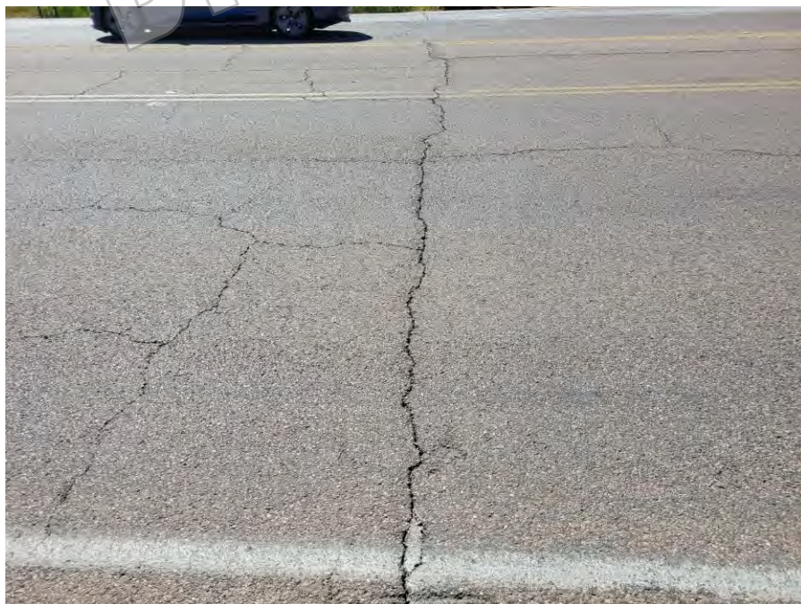
Photograph 2: Typical block cracking.
