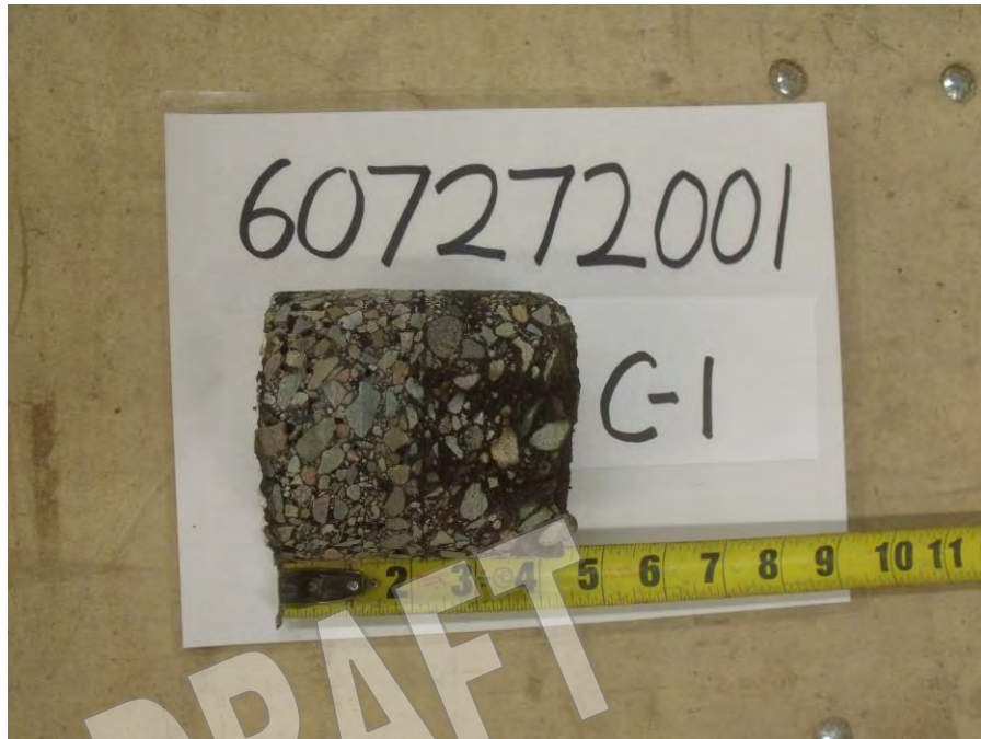
Photograph 7: Core Location C-1, asphaltic concrete thickness approximately 4.5 inches. Approximately 6 inches of aggregate base at C-1
