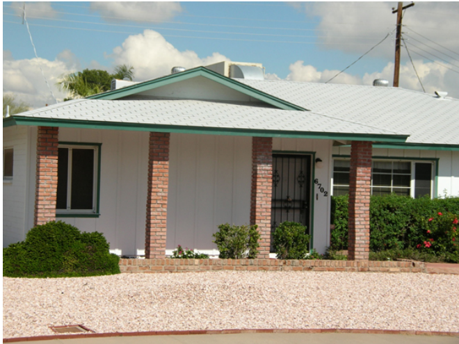
Changing the wooden posts on the porch to wider red-brick columns is not appropriate because it changes the scale and appearance of the columns.
