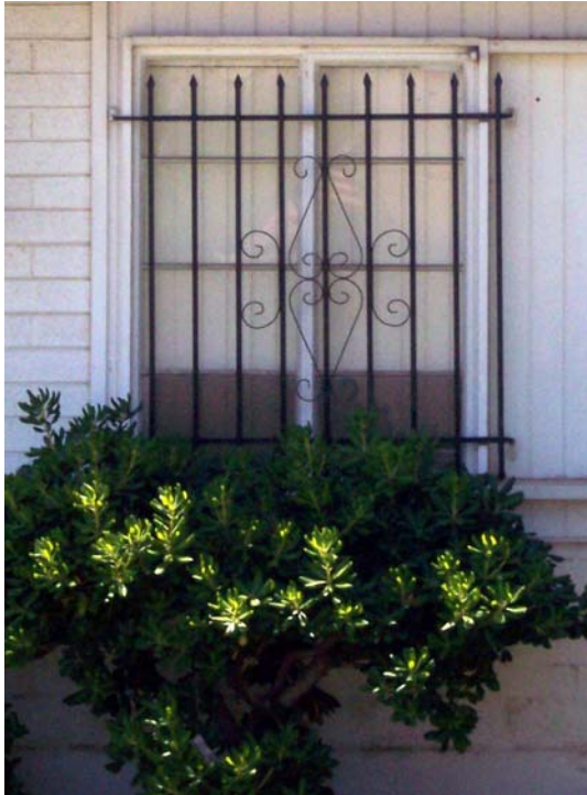
Metal security grilles detract from the original appearance of the windows.
