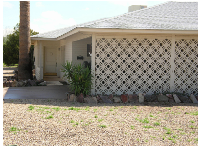
The use of decorative screen blocks on the side of this carport was a typical detail from the Ranch style era.
