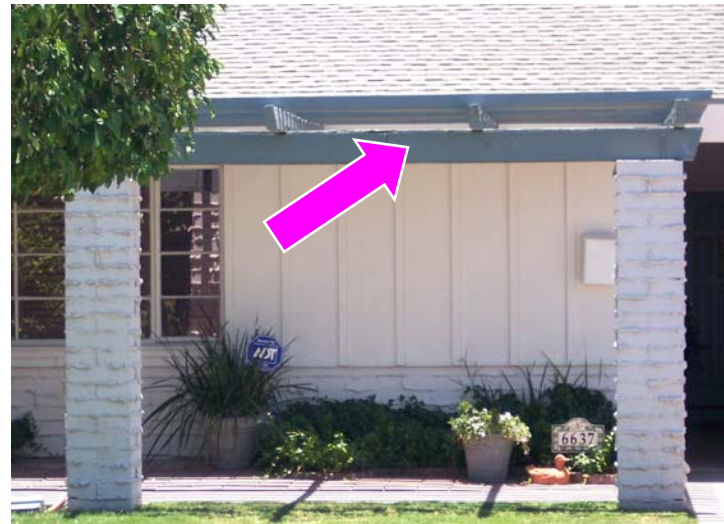
Installing a flat patio/porch roof out of heavy timbers on heavy columns is not recommended. The roof and column materials have a different scale and texture than the historic building materials.
