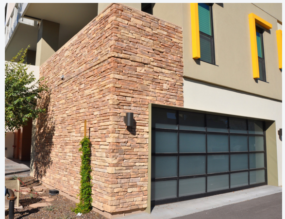
DISCOURAGED - Stacked stone abruptly transitions to smooth stucco, with no horizontal change in wall plane, highlighting the simulated nature of the material.
