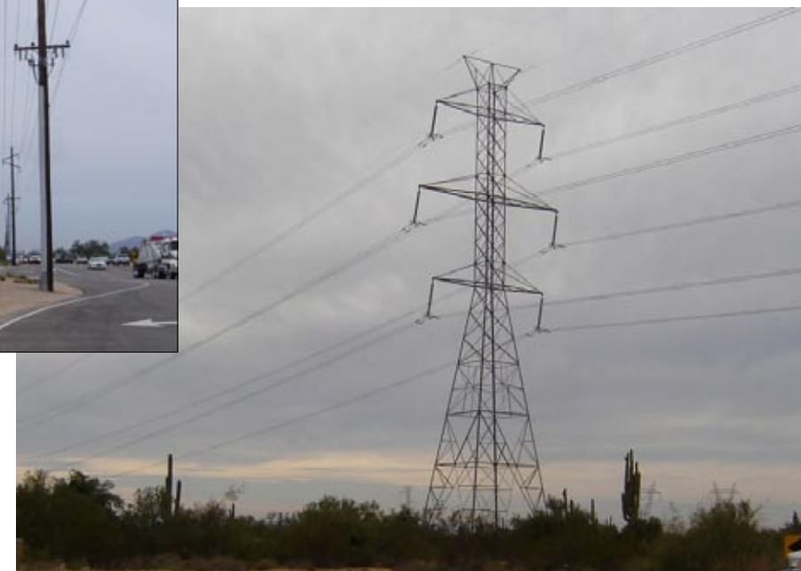
High voltage transmission towers and lines cross the corridor in multiple locations
