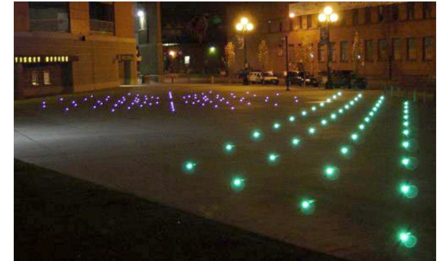
In-ground accent lighting - to be used in a limited manner
