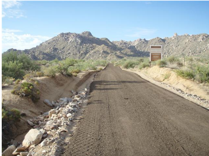
Recycled asphalt used to minimize dust on the road to Tom’s Thumb Trailhead in the Preserve
